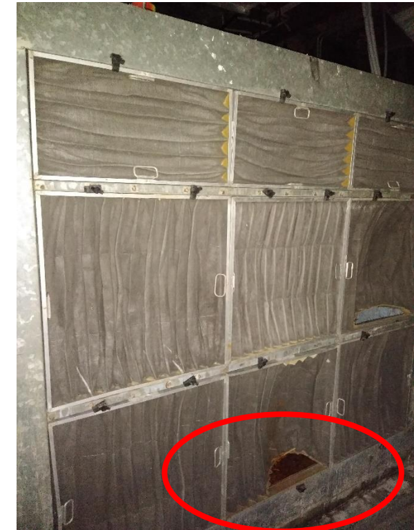
Poor maintenance of filtration systems
