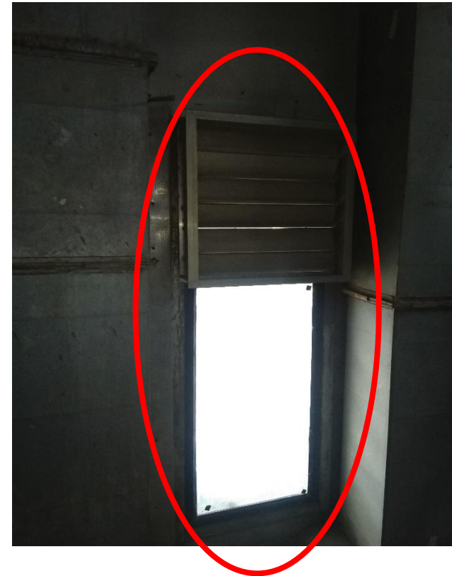
Closed outdoor air damper
